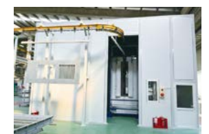
Powder coating facility that started operation in March 2022
