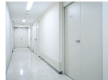
Fireproof steel door (Sanwa Shutter)
