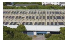
Solar power generation equipment at Shanghai Baosteel-Sanwa Door (China)
