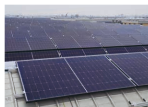
Solar power generation equipment at Novoferm Schievano (Italy)
