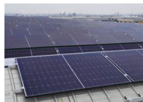
Solar power generation equipment at Novoferm Schievano (Italy)
