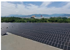
Solar power generation equipment at the Sanwa Shutter Corporation Kyushu Plant
